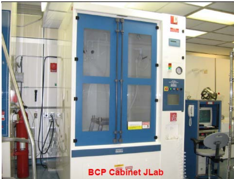
BCP Cabinet at Jlab, USA
